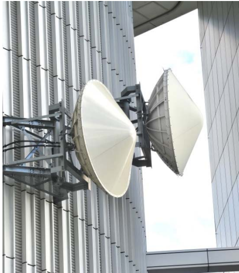
Microwave data backhaul
